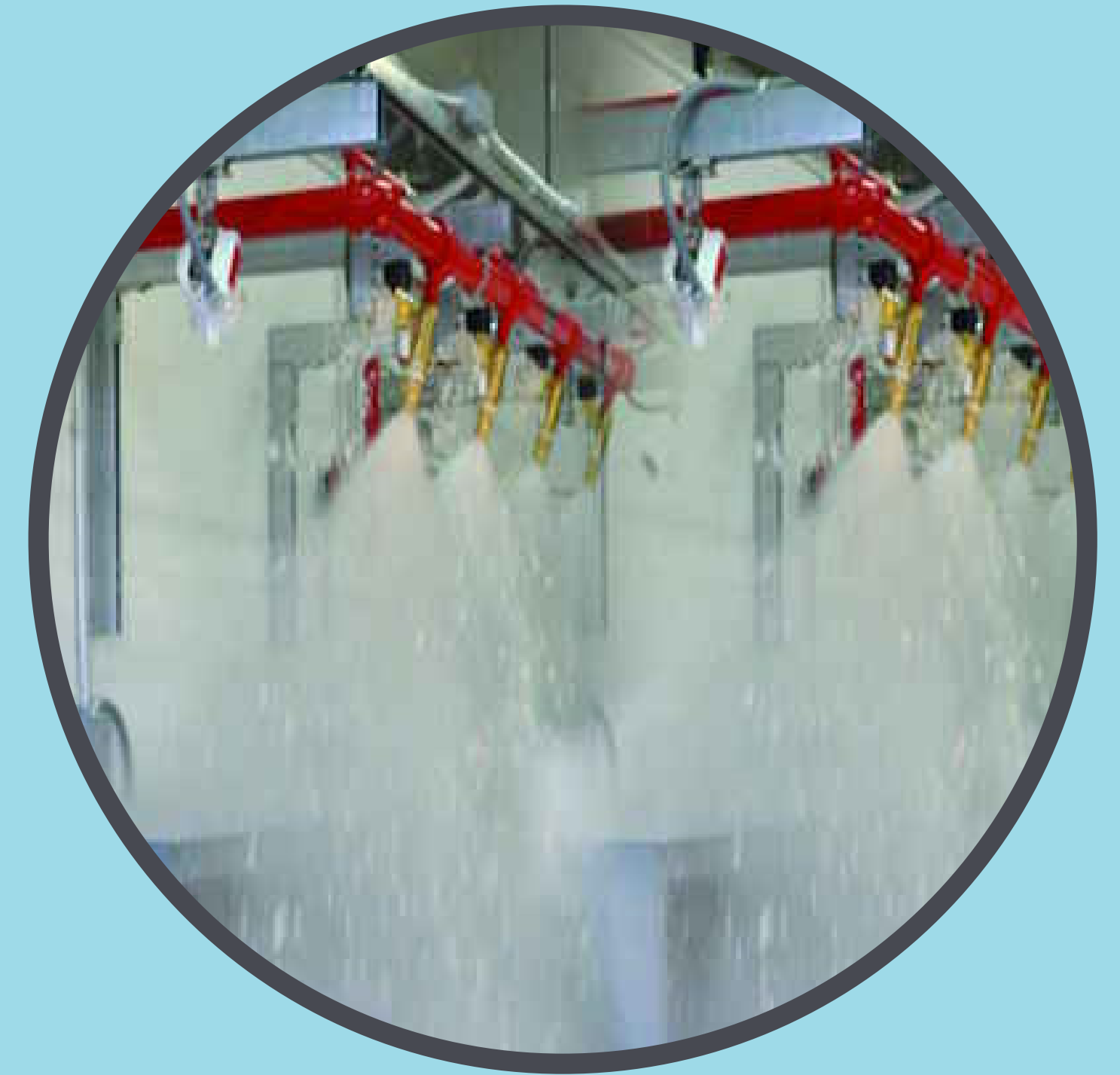
WATER CURTAIN SYSTEM
