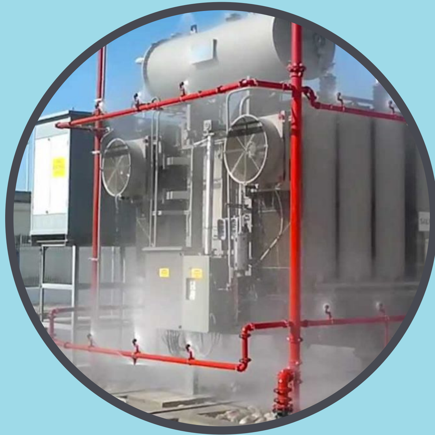
HIGH VELOCITY WATER SPRAY SYSTEM (HVWS)
